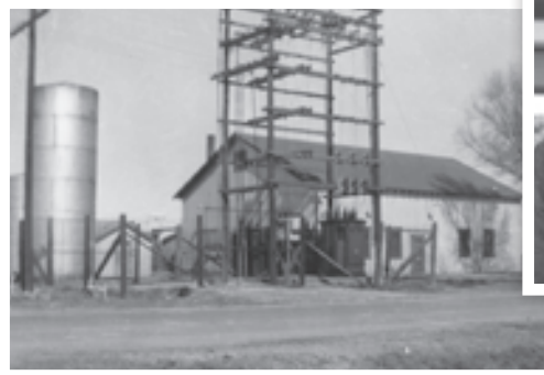
Avenue D Plant
